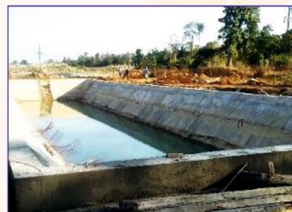
Permanent Settling Tank
