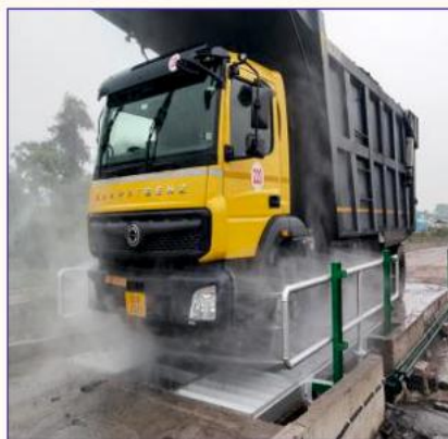
Wheel washing facility
